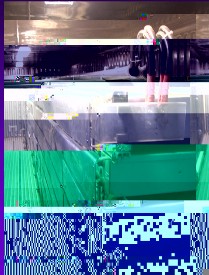
Batteries 3MW Total
